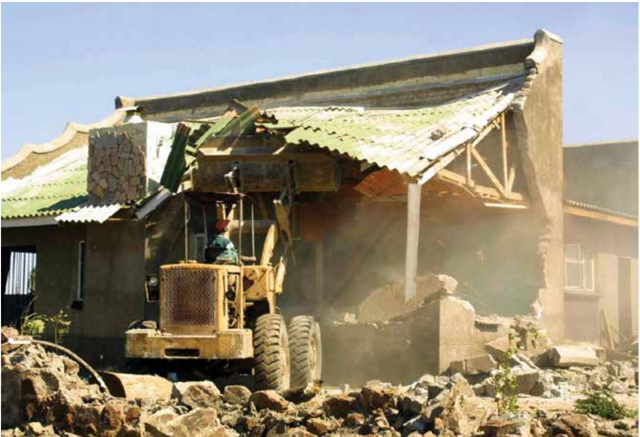
Zimbabwe's government clean-up campaign, Operation Murambatsvina (Clean the Filth), displaced thousands of poor urbanites.
